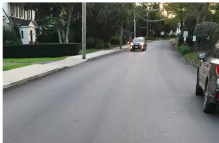
Absence of yellow centre line
